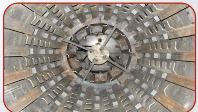
Inside Dryer Drum
